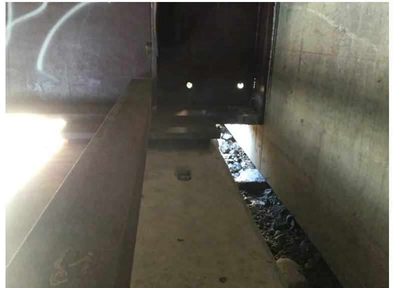
No damage noted to girders where they were drug through river
