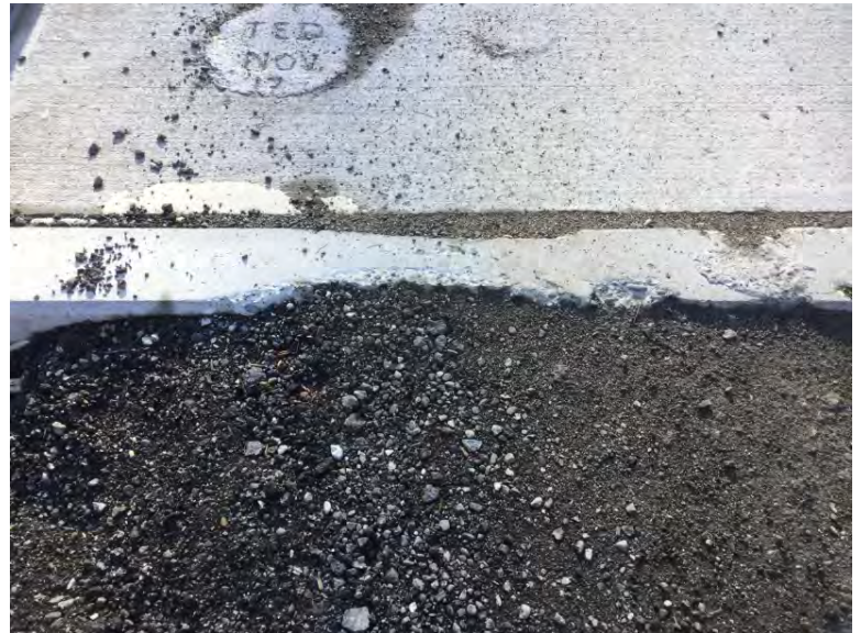
Damage to top of ballast wall right bank
