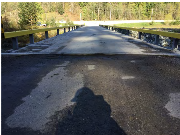
Left approach could use additional surfacing
