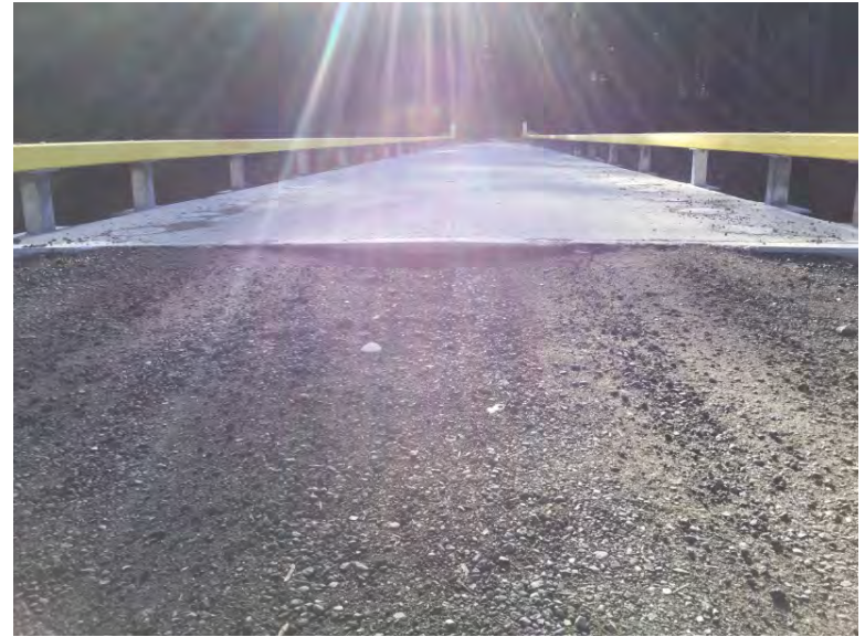
Right approach could use additional surfacing
