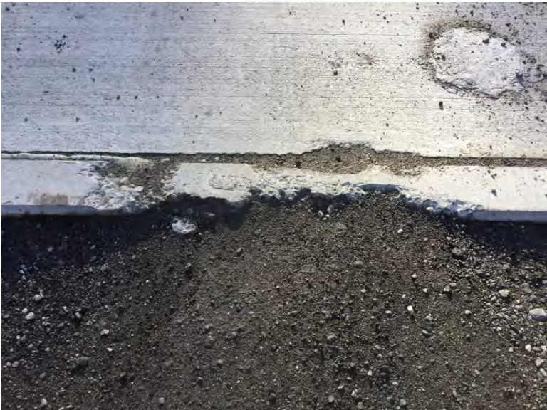
Damage to top of ballast wall on right bank
